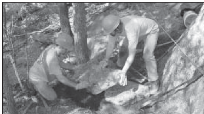
John Kahle and John Hiller set a staircase rock on the new trail around Eagle Cliff. Photo by Eric Morse.
