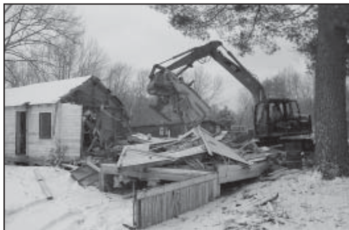
Randy Eastman was contracted by SLA to demolish old motel cabins on the recently acquired Harrison property, Photo by Eric Morse.
