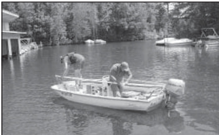
Brett Durham (SLA Ecological Manager) and Jeremy Mears (Plymouth State University Biology Intern) install a 10 foot square pipe to measure the injection of lime slurry at Kimbell Marina. Photo by Eric Morse.
