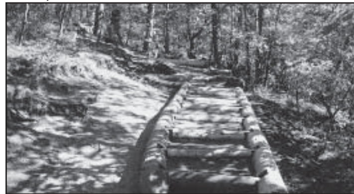
After... A crib staircase was constructed to prevent further erosion. Photo by Eric Morse.
