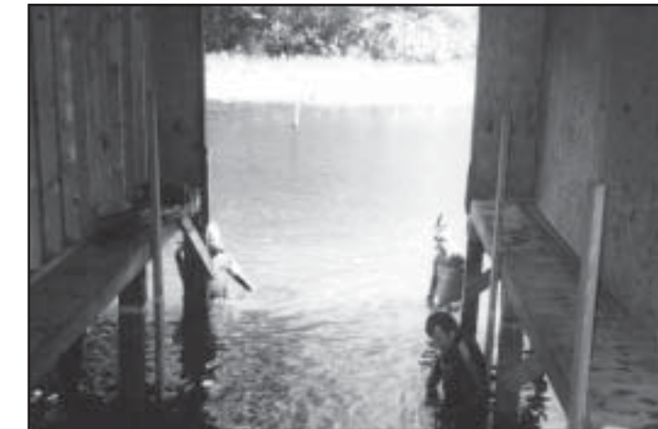
David Graham Wolf, Eric Morse and Chris Devine install a bottom barrier in a boathouse on the Squam Channel to prevent the spread of Variable Milfoil. Photo by Tom Morse.
