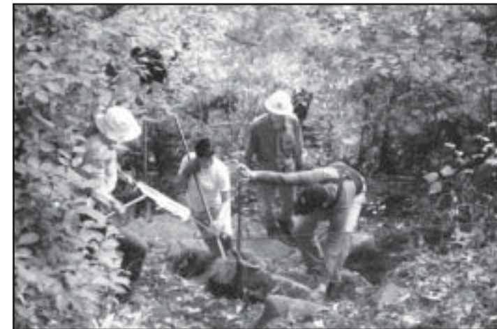
The SLA Trail Crew moves a large rock on the Crawford-Ridgepole Trail with a GripHoist winch. Photo by Eric Morse.
