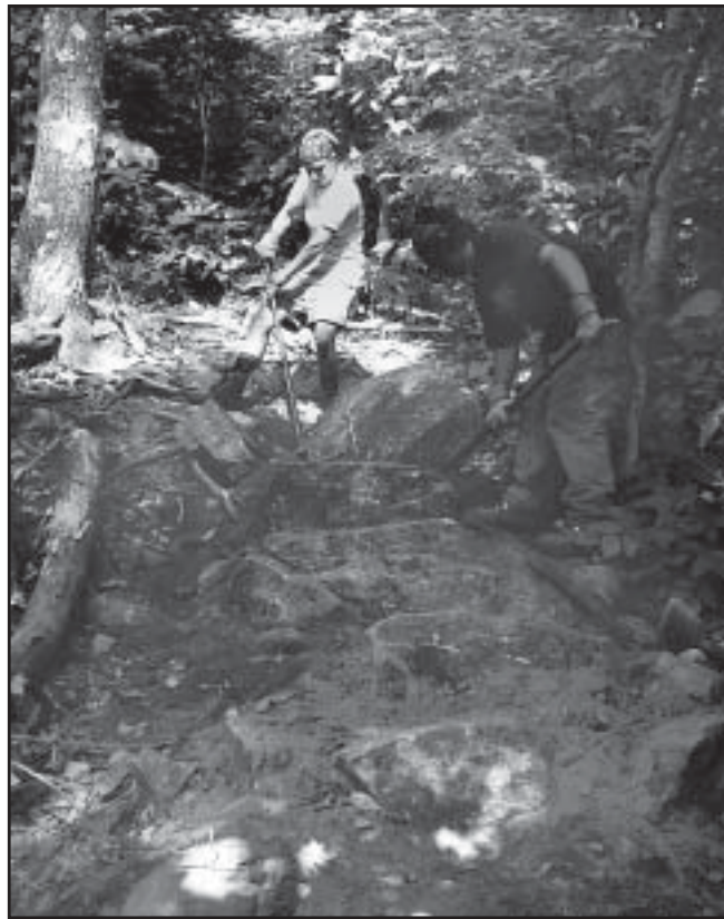
Jeanette Prost and Ben Gaglioti build a rock staircase on a steep section of the Mt. Percival Trail. Photo by Eric Morse.
