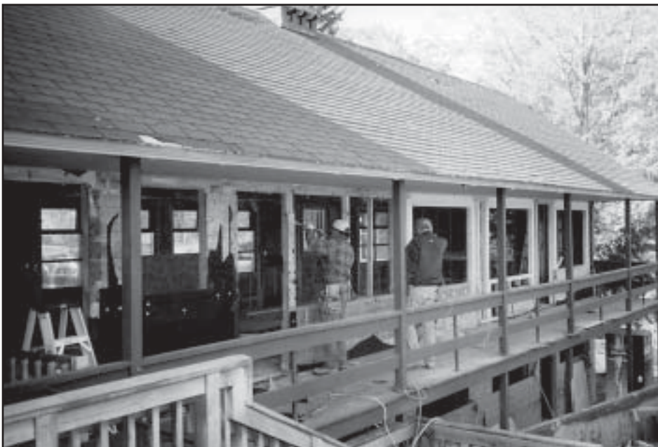
The SLA Resource Center renovation began on October 17th. Photo by Eric Morse.
