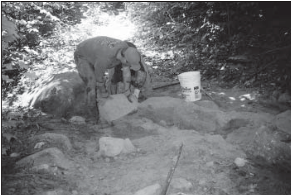
SLA Trail Crew members build a rock waterbar to provide drainage on the Mt. Percival Trail. Photo by Eric Morse.
