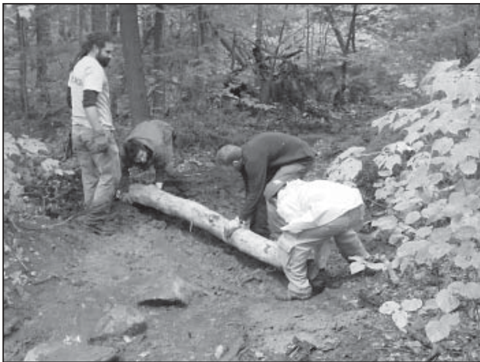
The SLA Trail Crew (Nelson Bruni, Brandon Kielbasa, David Morrill, Bob Struble and Atticus Doman) install a log waterbar on the Mt. Morgan Trail. Photo by Eric Morse.
